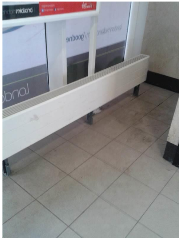
RH Low Level Radiator with concourse tiles
