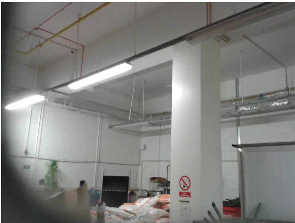
High level pipework in former parcels office – Note support column rising through slab
