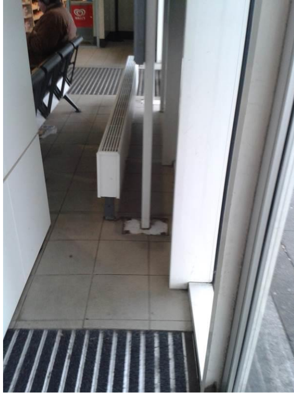
Centre LH Low Level Radiator with concourse tiles & well mat
