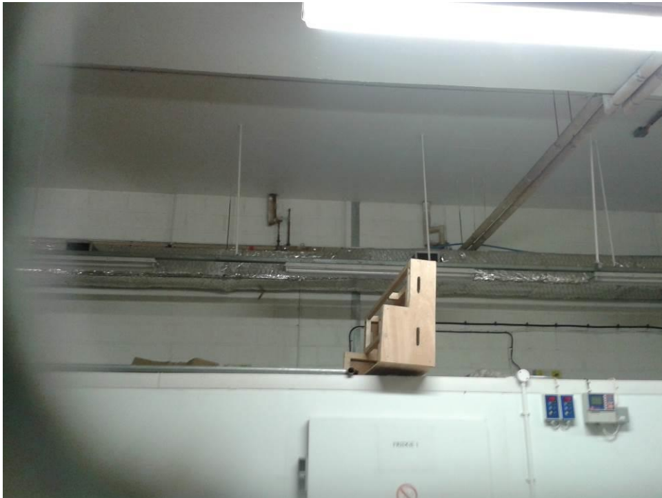
High level pipework in former parcels office – note pipework rising through floor slab
